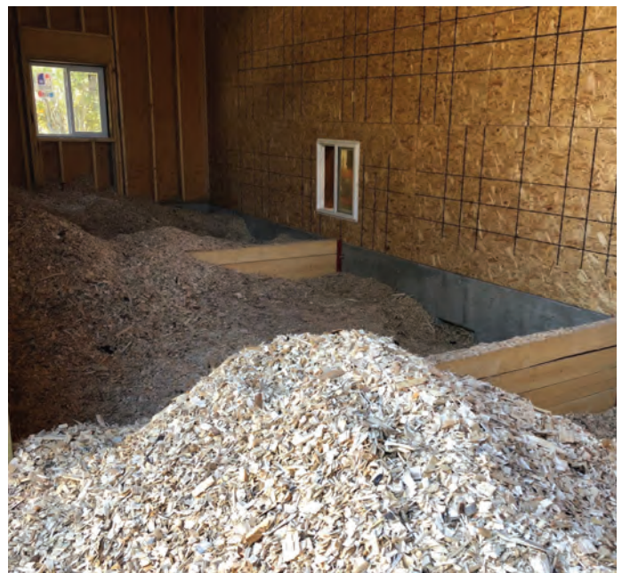
Wood chips are used as fuel in biomass boilers to heat ten community buildings.
