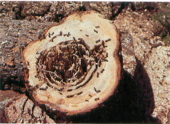
Fig. 5-1. Damage caused by carpenter ants.
